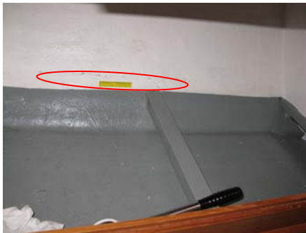
Visual hairline crack at the upper end of the tank-tabbing.
