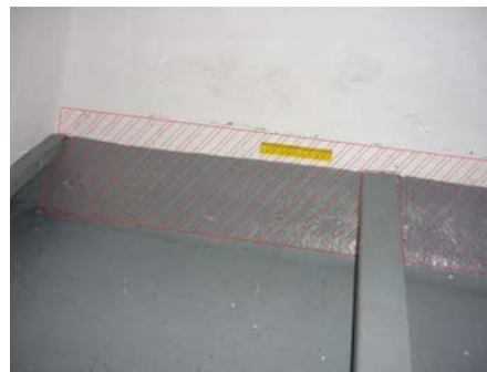
Actual area affected by debonding as indicated by Ultrasonic Flaw Detection
